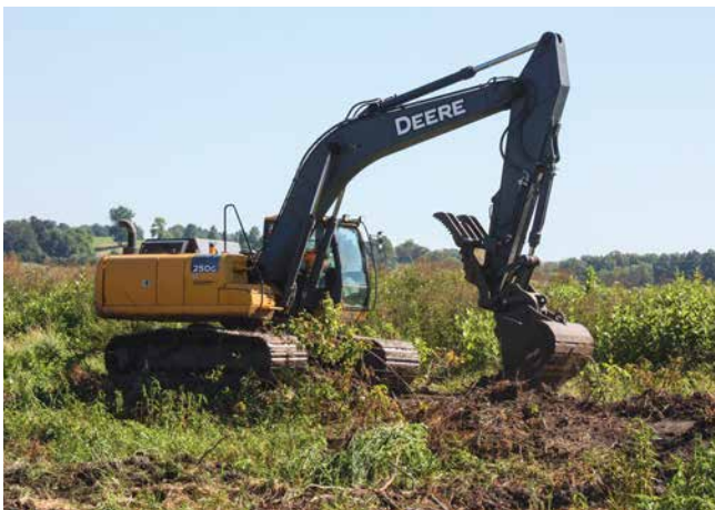
Figure 49: Track hoe. Typically used for pipe installation or other targeted excavations, here it is being used to downgrade an existing levee where access by more traditional equipment was prohibited by wetness.
