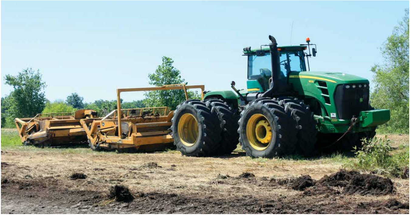
Figure 48: Tractor pulling a scraper. Today, this is the go-to earthmoving method used in wetland restorations because it allows for borrow material to be obtained from across the entire project.
