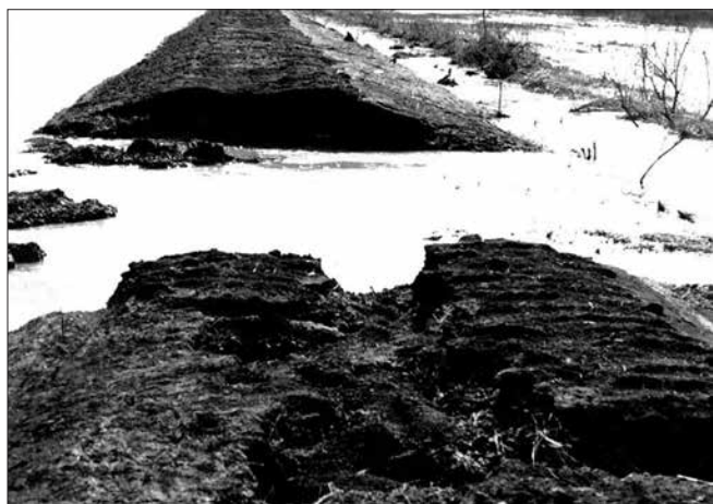
Figure 24: Wetland berm damaged by flooding soon after it was built.
