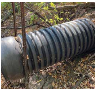
Figure 41: Corrugated plastic pipe (N12) installed in a berm. Buoyancy is an issue with this pipe due to the hollow corrugations. This pipe has been strapped between two posts to prevent floating.
