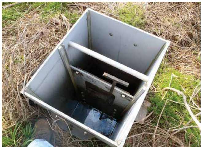
Figure 32a: Inline PVC type WCSs are popular choices for water level management. This one is fitted with an internal flap gate which occupies the top board position.
