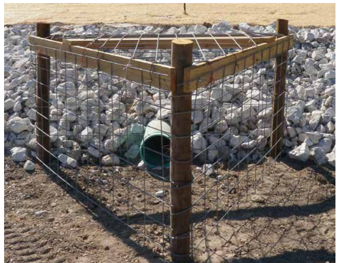
Figure 42: This constructed trash guard is designed to prevent debris and animal activity from obstructing the WCS and pipe.
