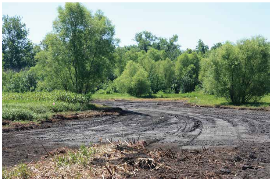
Figure 31b: Recently constructed creative borrow. Note how the layout weaves through existing woody cover to provide deep water next to willows.
