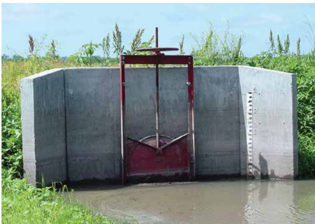
Figure 37: A screw gate mounted to a concrete headwall.
